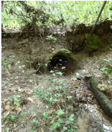
Photo 98. Inflow culvert that routes water from IFAS property into Wetland X within the Project Site (GPS 1755).
