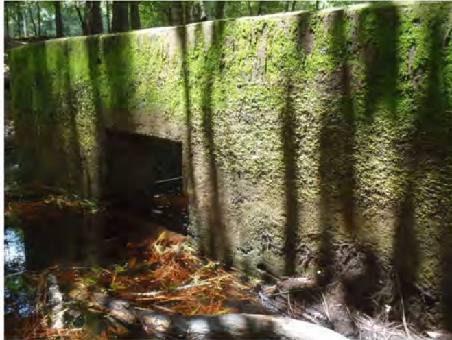
Photo 11. Upstream view of the east side of the Blues Creek overflow structure (GPS 820).
