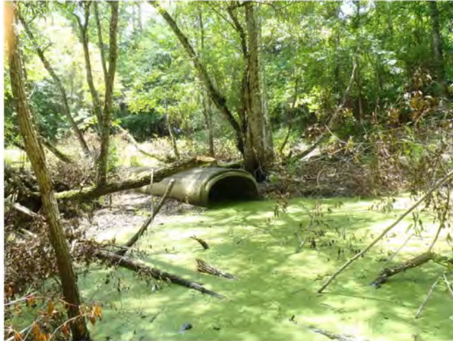
Photo 13. Pipe west of spillway within downstream area of where pipe discharges into Blues Creek Excavated Wetland (GPS 820).
