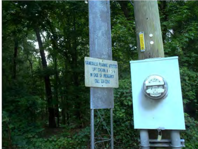
Photo 61. GRU sign at lift station (GPS 1272).
