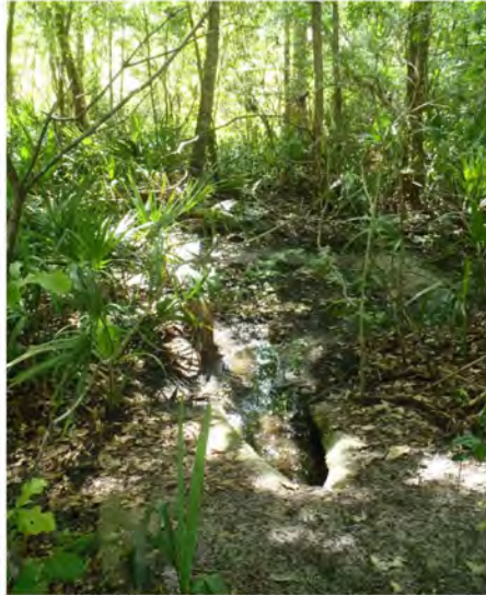
Photo 53. Stormwater inflow (GPS 1178).
