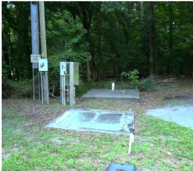
Photo 60. Lift station (GPS 1272).
