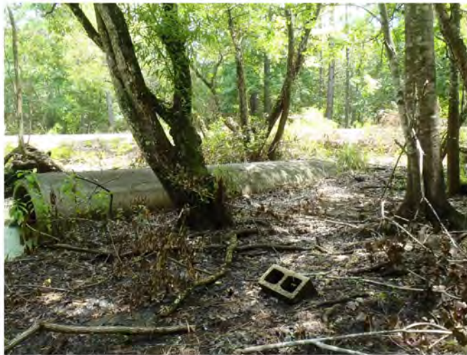
Photo 12. Pipe west of spillway on downstream side (GPS 820).
