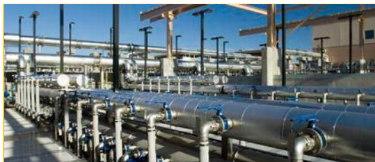
Kyrene Water Reclamation Facility project, a 4.5-MGD expansion of the existing conventional WRF to a 9 MGD state-of-the-art membrane and UV technology plant.
