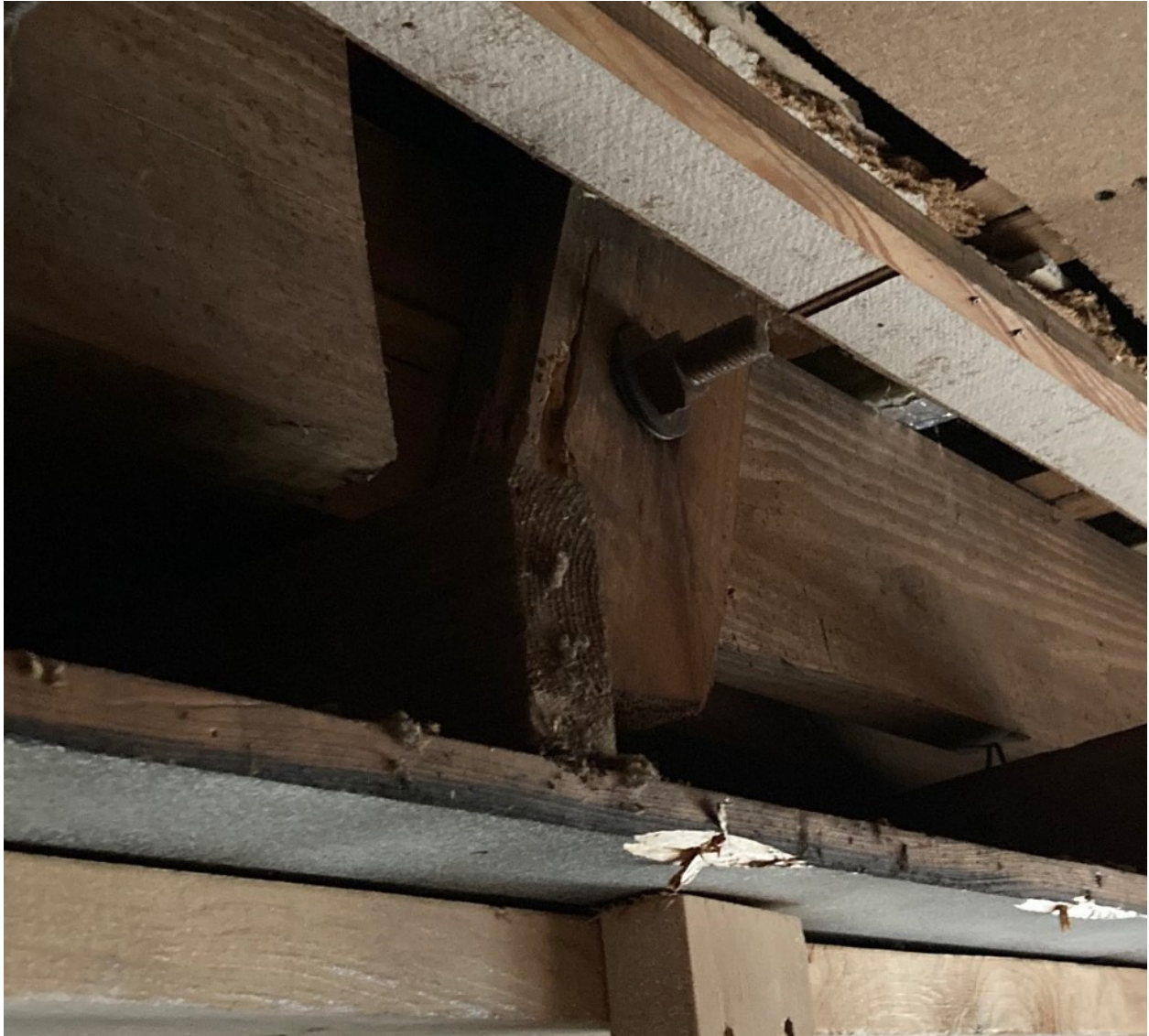
Figure 12. Termite damage extending into connection
