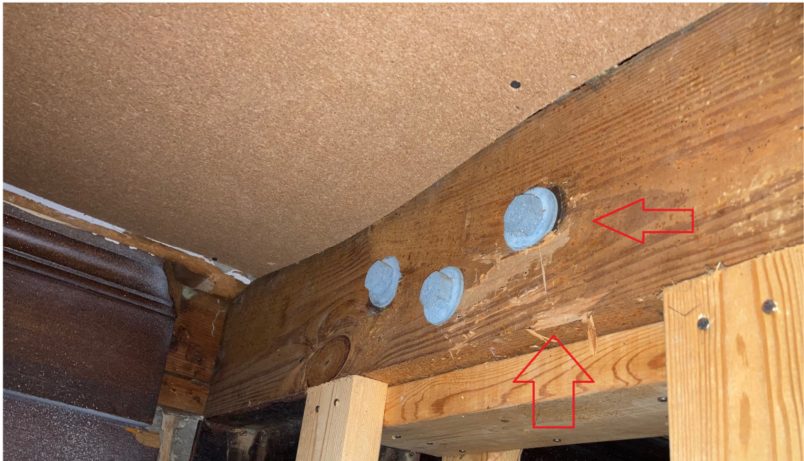
Figure 11. Termite damage to truss chord, including under bolt heads
