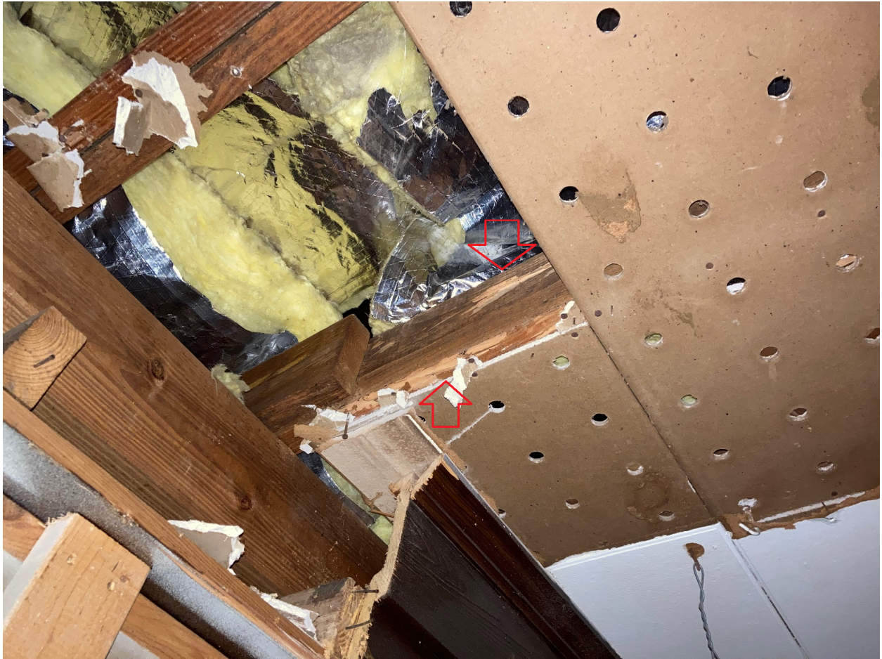
Figure 5. Termite damage to ceiling joist
