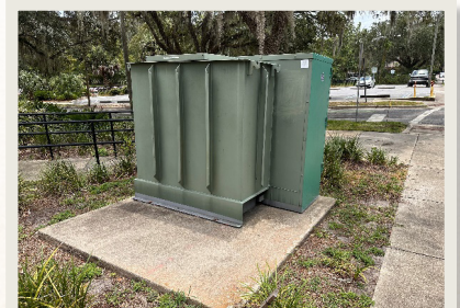
Figure 11: Existing GRU Transformer
