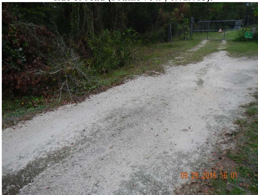
Photo 439. View of Physical Feature: Culvert at GPS locations 8101-8102. View is of north side of culvert (Frame 7650; 09/29/15).
