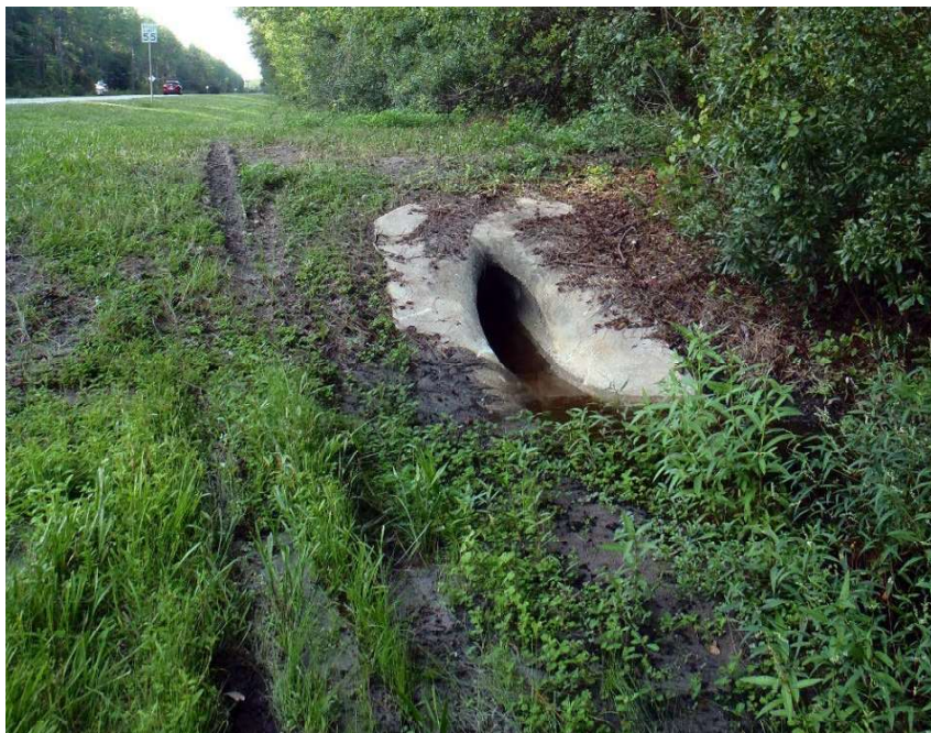
Photo 239. View of Physical Feature: Culvert located on east side of road as seen looking north from GPS location 5203 (Frame 1931; 09/02/15).
