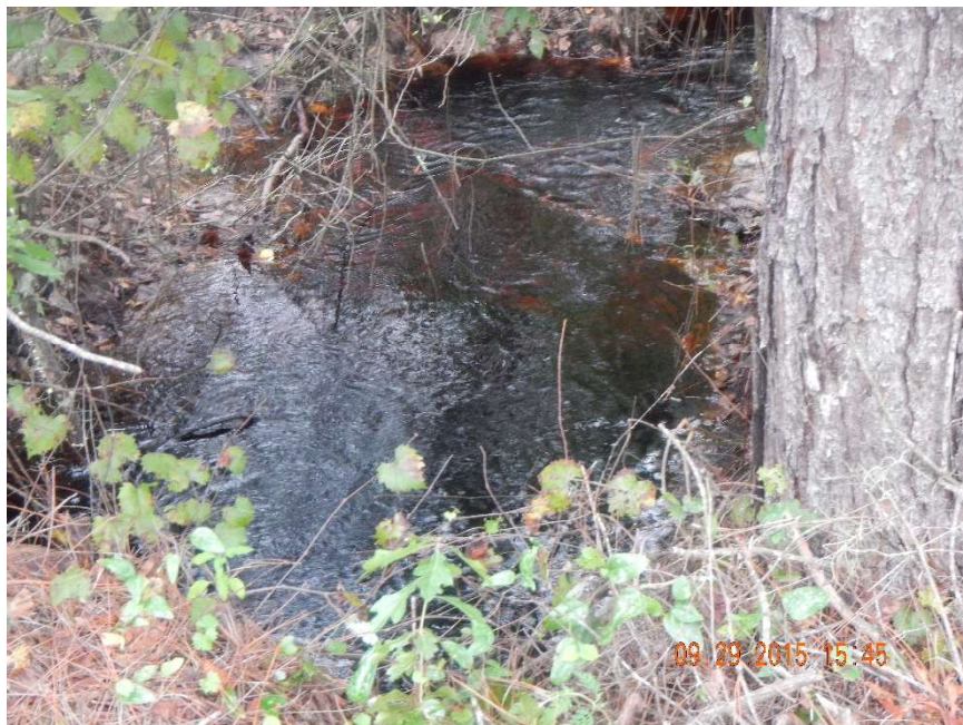
Photo 438. View of flow at Physical Feature: Culvert at GPS location 8100. Flow is to north on north side of road (Frame 7649; 09/29/15).
