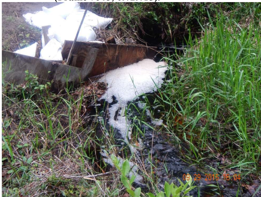
Photo 437. View of flow at Physical Feature: Culvert at GPS location 8099. View is to north on south side of road. Flow has eroded south side of road (Frame 7652; 09/29/15).
