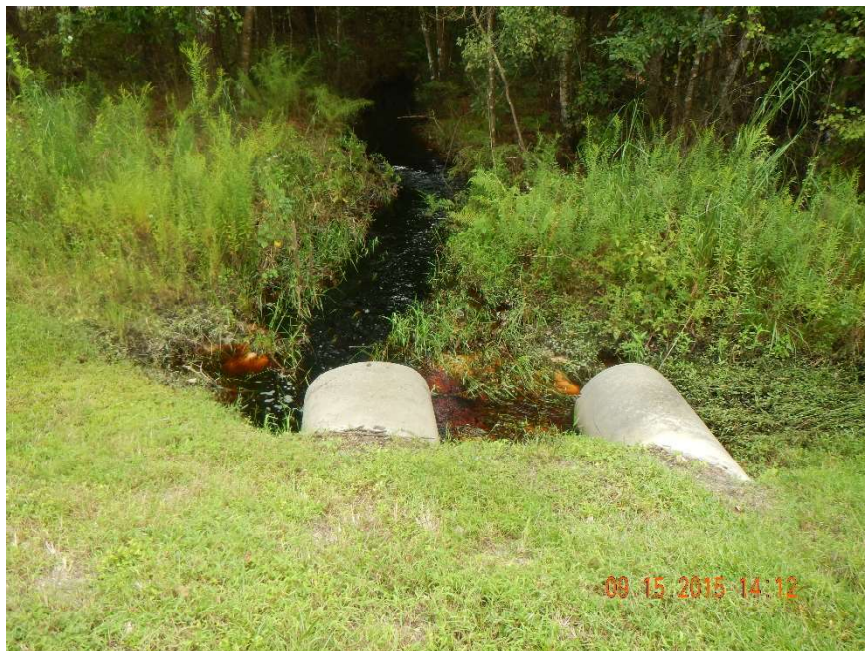
Photo 360. View to south (upstream) of culverts located in Rocky Creek at GPS location 9841 (Frame 7490; 09/15/15).
