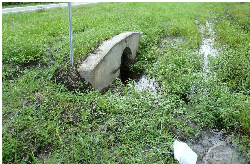
Photo 217. View of Physical Feature: Culvert located on west side of road as seen at GPS location 1696 (Frame 1892; 08/31/15).
