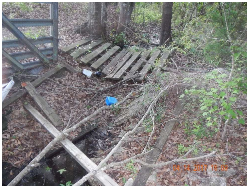
Photo 536. View of collapsed culvert and roadway at offsite drainage divide as seen looking west from GPS location 10304 (Frame 1451; 04/14/17).
