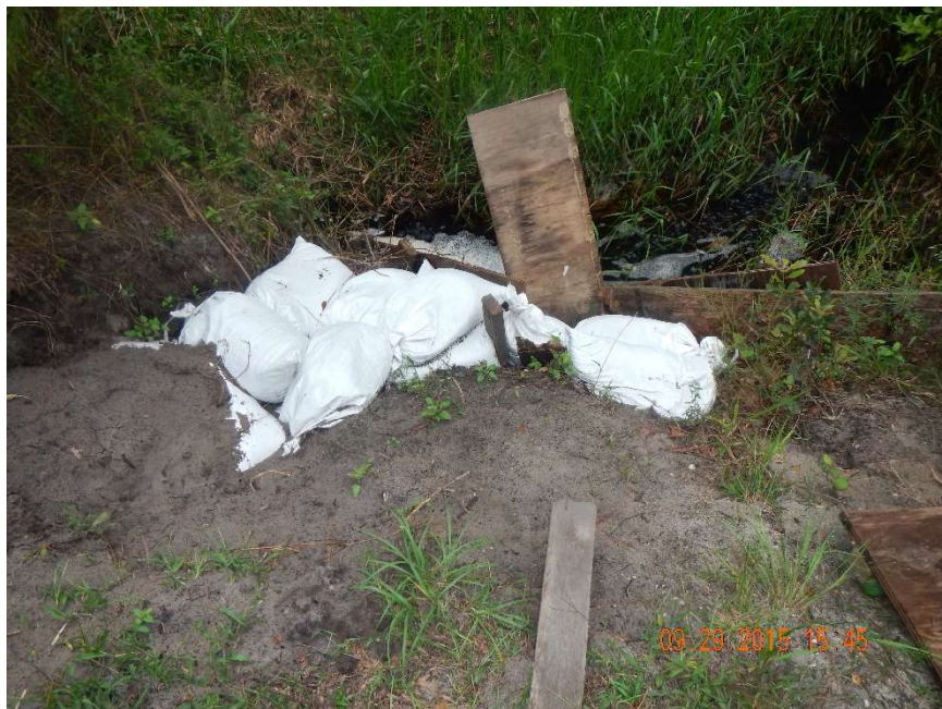
Photo 436. View of eroded Physical Feature: Culvert as seen looking south from GPS location 8099 (Frame 7648; 09/29/15).
