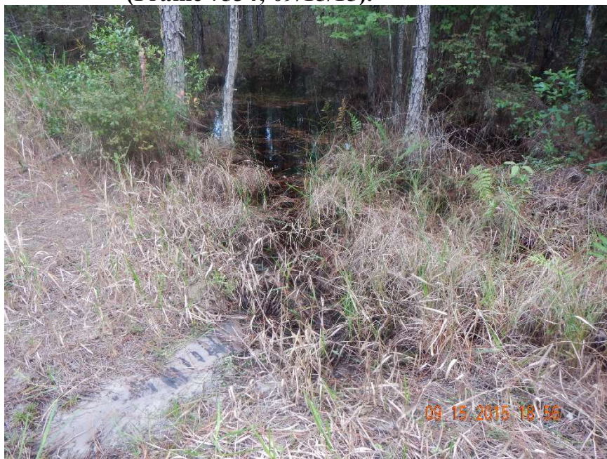
Photo 399. View of Physical Feature: Culvert as seen looking north (downstream) from GPS location 7497 (Frame 7535; 09/15/15).
