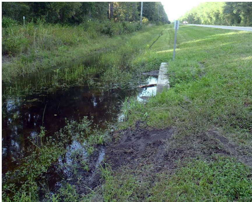
Photo 237. View of Physical Feature: Culvert located on west side of road as seen looking north from GPS location 5201 (Frame 1929; 09/02/15).
