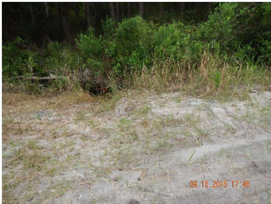
Photo 382. View of north end of Physical Feature: Culvert that runs north from GPS location 7403 to 7404 and routes water in this direction (Frame 7516; 09/15/15).
