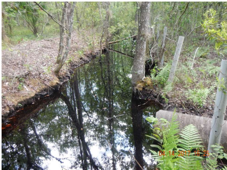
Photo 522. View of culvert located in old ditch that intercepts deeper, more recent excavation at GPS location 10184 (Frame 1431; 04/14/17).
