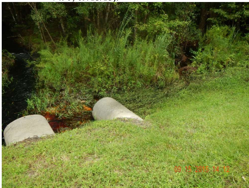
Photo 361. View to south (upstream) of culverts located in Rocky Creek at GPS location 9841 (Frame 7491; 09/15/15).
