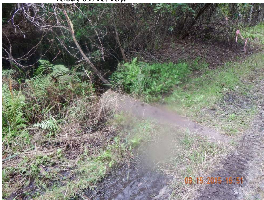
Photo 373. View of Physical Feature: Culvert as seen looking at east end (downstream) of culvert at GPS location 7360 (Frame 7504; 09/15/15).
