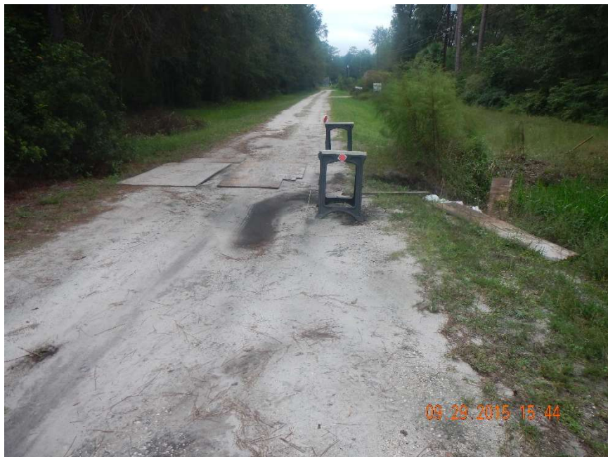
Photo 434. View of eroded Physical Feature: Culvert as seen looking east from GPS locations 8099-8100 (Frame 7646; 09/29/15).
