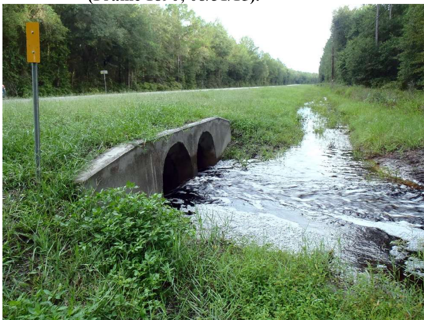
Photo 216. View of Physical Feature: Culvert located on west side of road as seen at GPS location 1694 (Frame 1891; 08/31/15).
