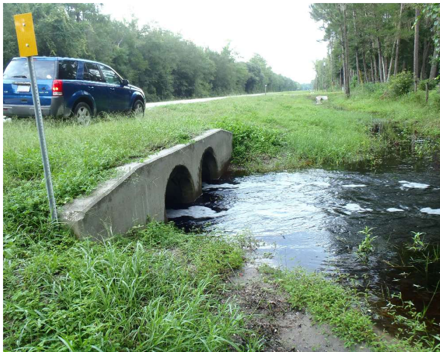
Photo 215. View of Physical Feature: Culvert located on east side of road as seen at GPS location 1693 (Frame 1890; 08/31/15).
