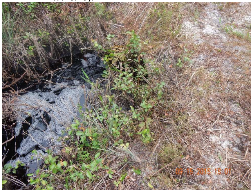
Photo 387. View of flow-way at west end of Physical Feature: Culvert located in gas line right-of-way at GPS location 7421 (Frame 7521; 09/15/15).
