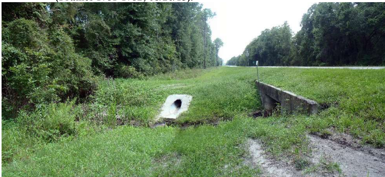
Photo 144. View of Physical Feature: Culvert as seen looking south from GPS location 1039 (Frames 1783-1784; 08/26/15).
