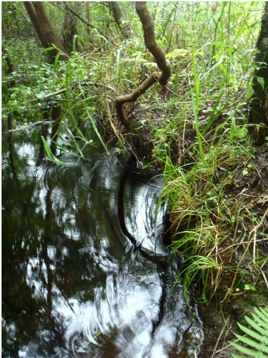
Photo 210. View of Physical Feature: Culvert located on south side of road at GPS location 1570 (Frame 1881; 08/31/15).
