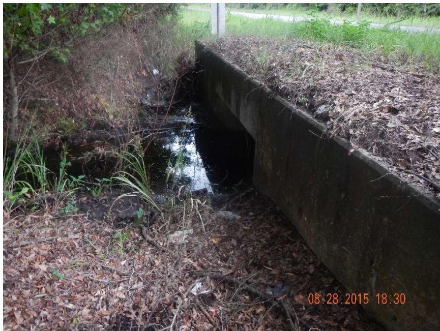
Photo 192. Rocky Creek: view to south of box culvert on east side CR 231 at GPS location 1516 (Frame 7407; 08/28/15).
