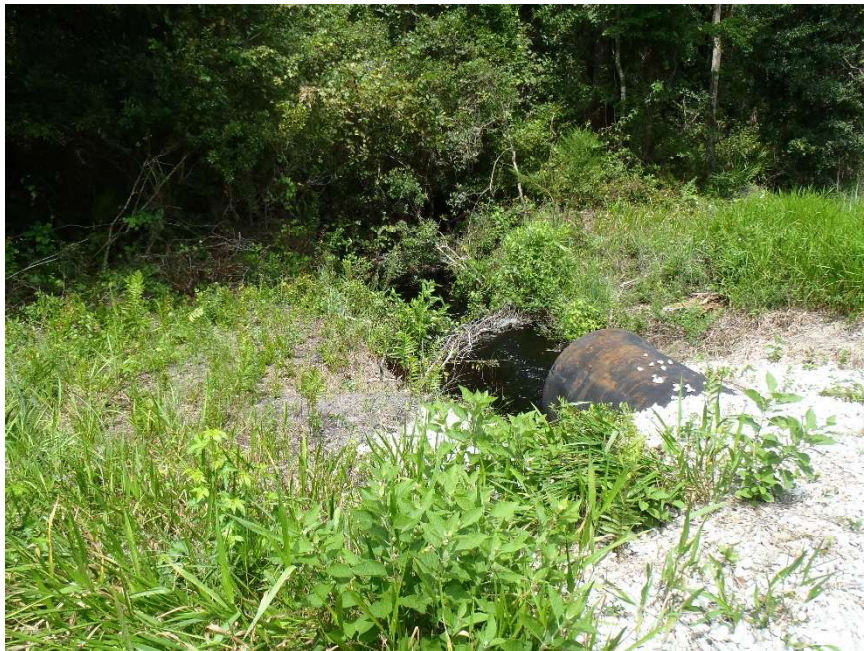
Photo 162. View of Physical Feature: Culvert located on north side of power line easement at GPS location 1176 (Frame 1815; 08/27/15).
