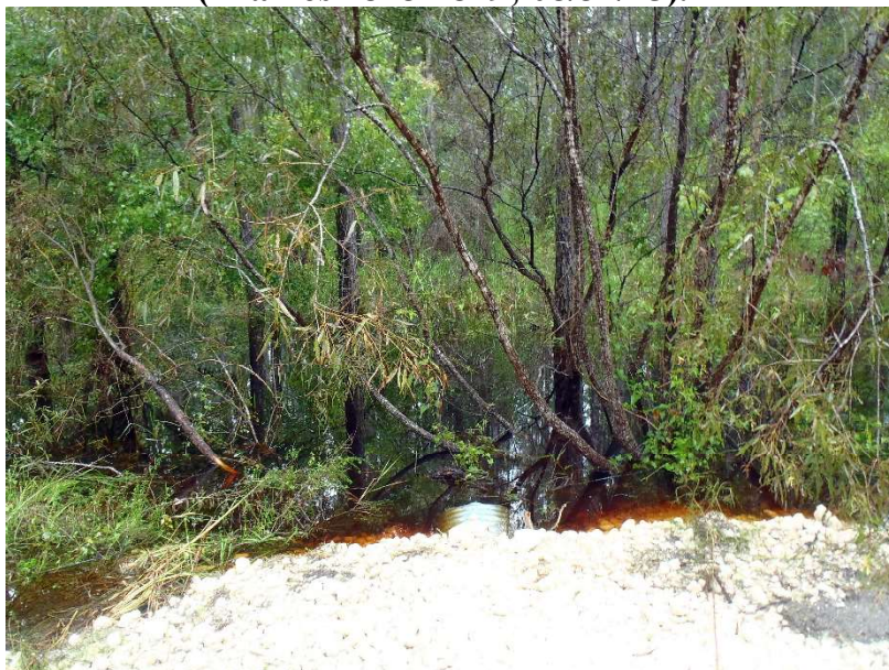
Photo 209. View of Physical Feature: Culvert located on north side of road at GPS location 1623 (Frame 1880; 08/31/15).
