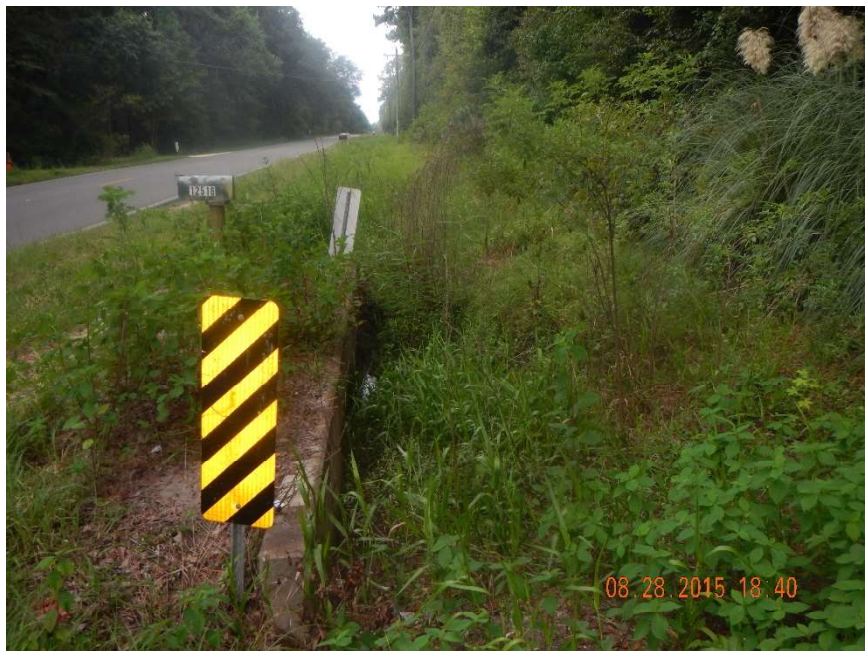
Photo 196. Rocky Creek: view to south of culvert at west side of CR 231 at GPS location 1517 (Frame 7412; 08/28/15).
