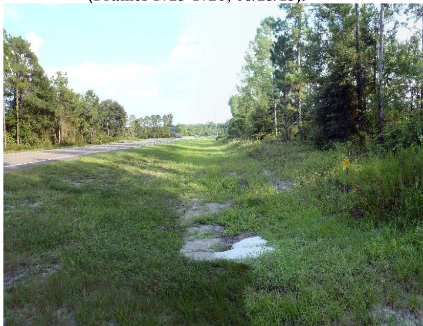
Photo 118. View of Physical Feature: Culvert as seen looking south from GPS location 2276 (Frames 1727-1728; 08/25/15).
