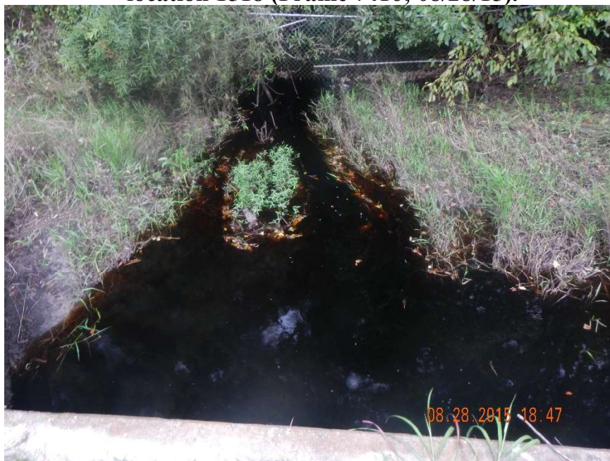
Photo 199. Rocky Creek: view to west (downstream) of major branch of Rocky Creek at culvert located at GPS location 1518 (Frame 7419; 08/28/15).
