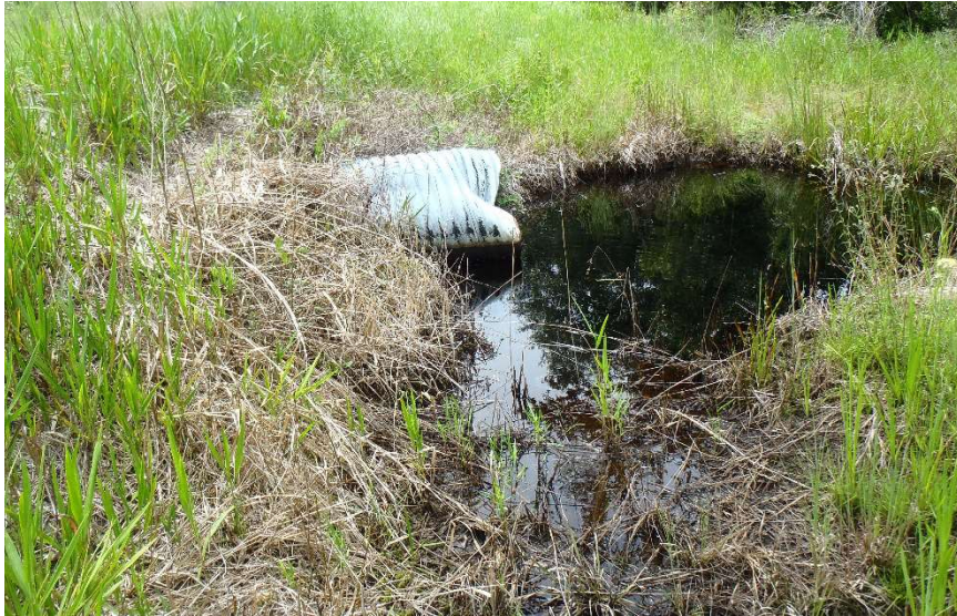
Photo 164. View of Physical Feature: Culvert located on north side of power line easement at GPS location 1177 (Frame 1817; 08/27/15).
