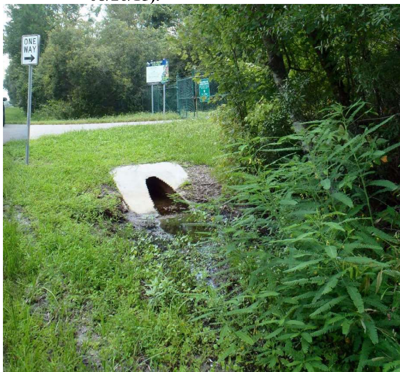
Photo 138. View of Physical Feature: Culvert as seen looking south from GPS location 1031 (Frames 1769-1670; 08/26/15).
