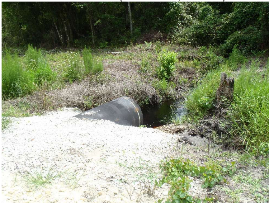
Photo 163. View of Physical Feature: Culvert located on south side of power line easement at GPS location 1176 (Frame 1816; 08/27/15).
