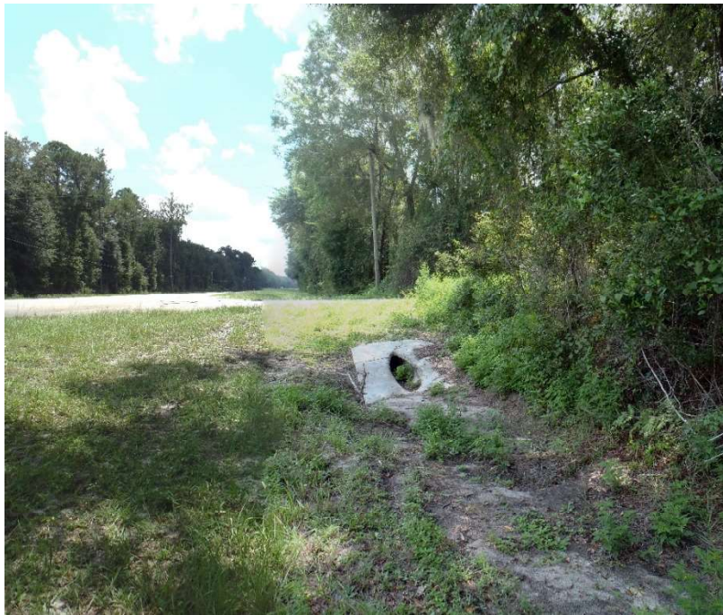
Photo 141. View of Physical Feature: Culvert as seen looking south from GPS location 1036 (Frames 1777-1778; 08/26/15).
