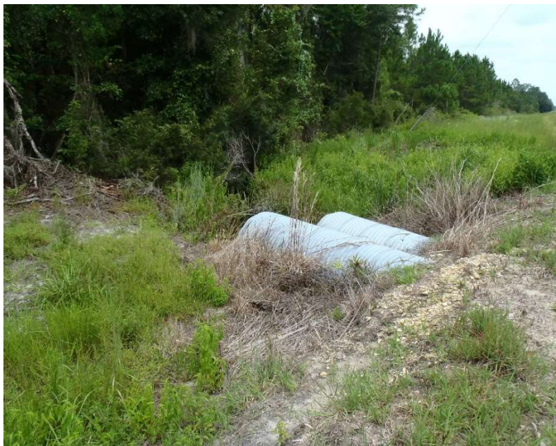
Photo 160. View of culverts on north side of power line easement within the Planted Pine-Mesic Pine Flatwoods located at GPS location 9000 (Frame 1813; 08/27/15).
