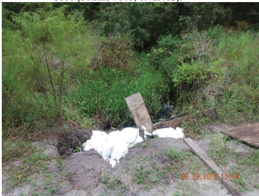
Photo 435. View of eroded Physical Feature: Culvert as seen looking north from GPS location 8100 (Frame 7647; 09/29/15).
