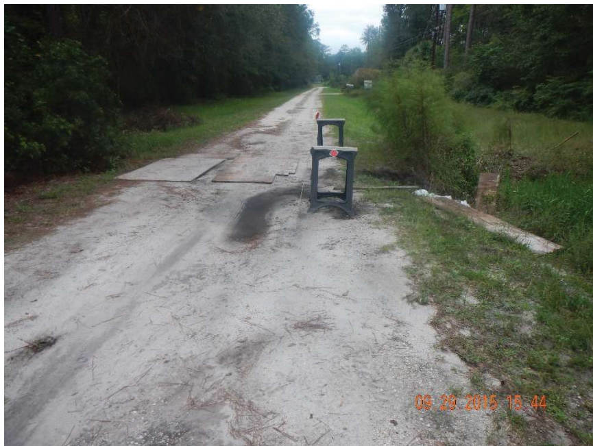
Photo 434. View of eroded Physical Feature: Culvert as seen looking east from GPS locations 8099-8100 (Frame 7646; 09/29/15).
