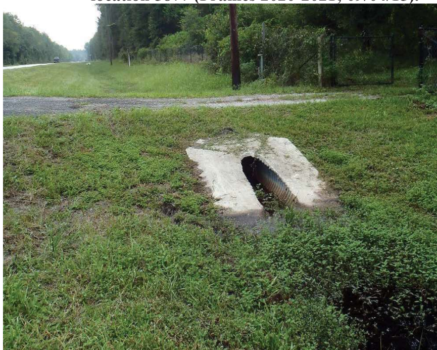
Photo 285. View of Physical Feature: Culvert as seen looking east from GPS location 5885 (Frame 2022; 09/04/15).
