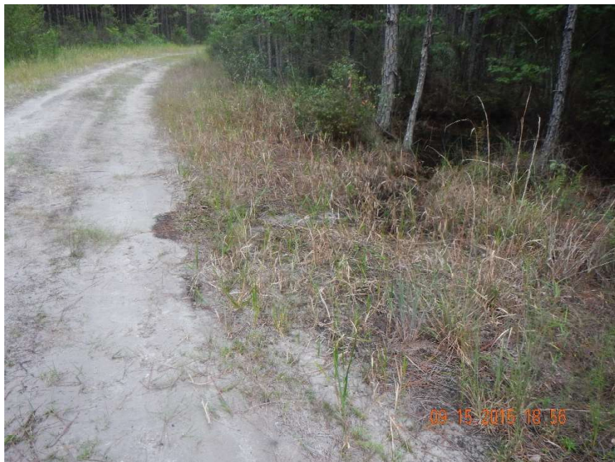
Photo 400. View of Physical Feature: Culvert as seen looking south (upstream) from GPS location 7497 (Frame 7536; 09/15/15).
