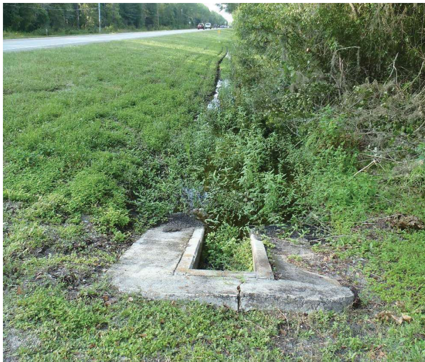
Photo 235. View of Physical Feature: Culvert located on east side of road as seen looking north from GPS location 5199 (Frame 1927; 09/02/15).
