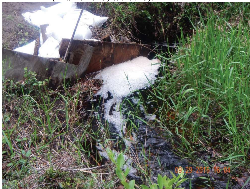
Photo 437. View of flow at Physical Feature: Culvert at GPS location 8099. View is to north on south side of road. Flow has eroded south side of road (Frame 7652; 09/29/15).
