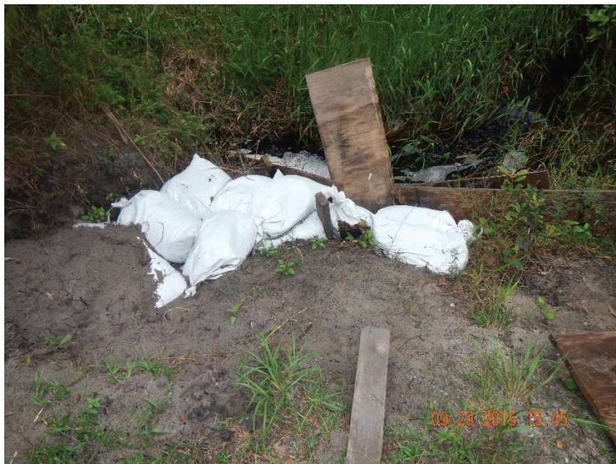
Photo 436. View of eroded Physical Feature: Culvert as seen looking south from GPS location 8099 (Frame 7648; 09/29/15).
