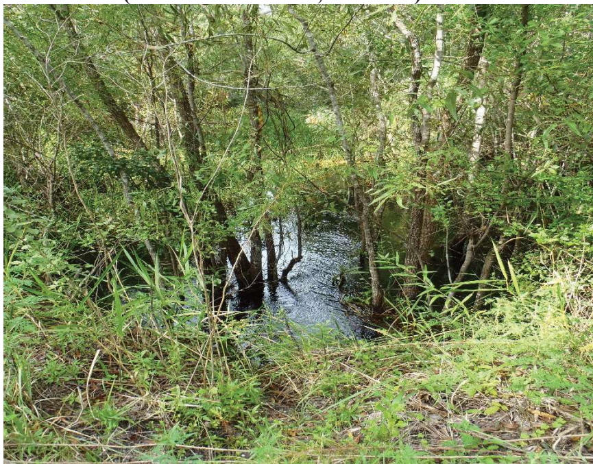
Photo 295. View of Physical Feature: Culvert as seen looking north from GPS location 6070 (Frame 2047; 09/08/15).
