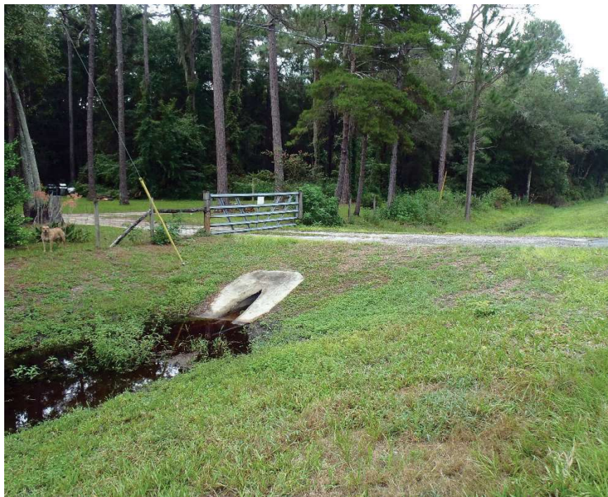
Photo 286. View of Physical Feature: Culvert as seen looking southeast from GPS location 5886 (Frame 2023; 09/04/15).
