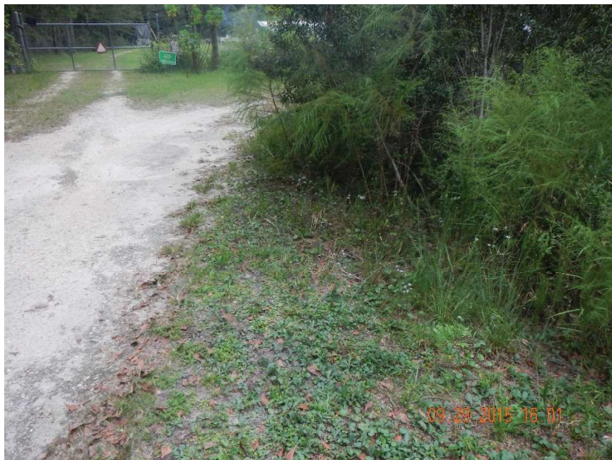
Photo 440. View of south side of Physical Feature: Culvert at GPS locations 8101-8102 (Frame 7651; 09/29/15).
