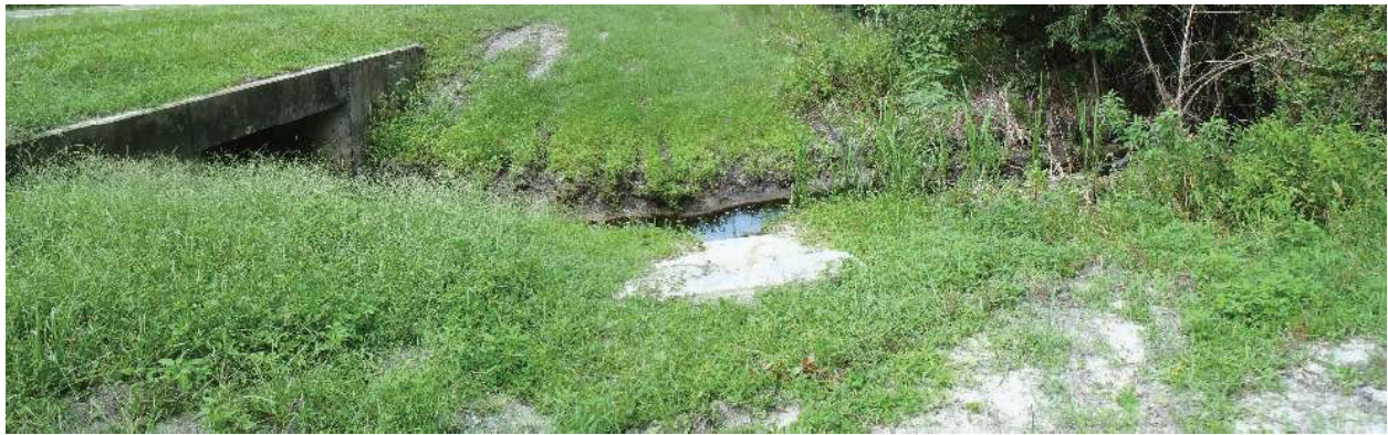
Photo 145. View of Physical Feature: Culvert as seen looking north from GPS location 1040 (Frames 1785-1786; 08/26/15).
