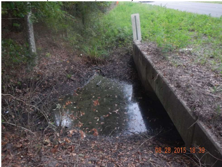
Photo 195. Rocky Creek: view to south of culverts located at GPS location 1517 on east side of CR 231 at GPS location 1517 (Frame 7411; 08/28/15).
