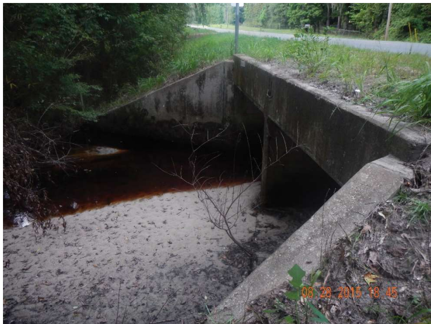
Photo 198. View to south of box culverts on east side (upstream) of CR 231 in Rocky Creek at GPS location 1518 (Frame 7416; 08/28/15).
