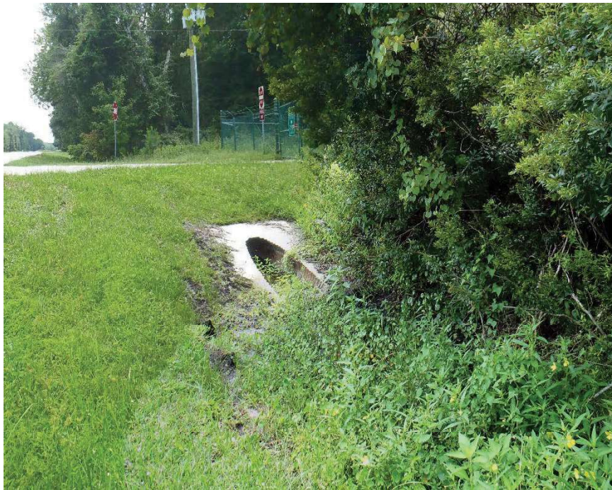
Photo 139. View of Physical Feature: Culvert as seen looking south from GPS location 1032 (Frames 1771-1772; 08/26/15).
