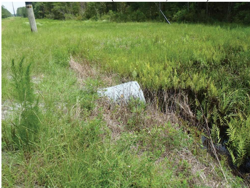
Photo 165. View of Physical Feature: Culvert located on south side of power line easement at GPS location 1177 (Frame 1818; 08/27/15).
