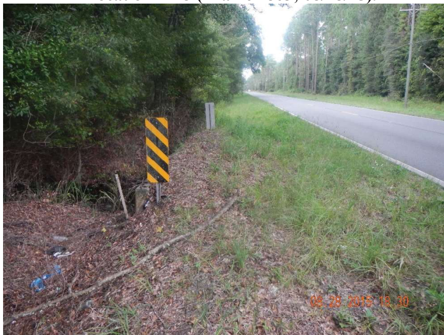
Photo 191. Rocky Creek: view to south of east side of culverts at CR 231 at GPS location 1516 (Frame 7406; 08/28/15).
