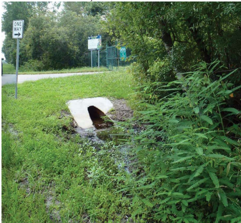
Photo 138. View of Physical Feature: Culvert as seen looking south from GPS location 1031 (Frames 1769-1670; 08/26/15).
