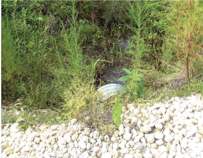
Photo 174. View of Physical Feature: Culvert located on north side of road at GPS location 1272 (Frame 1835; 08/27/15).
