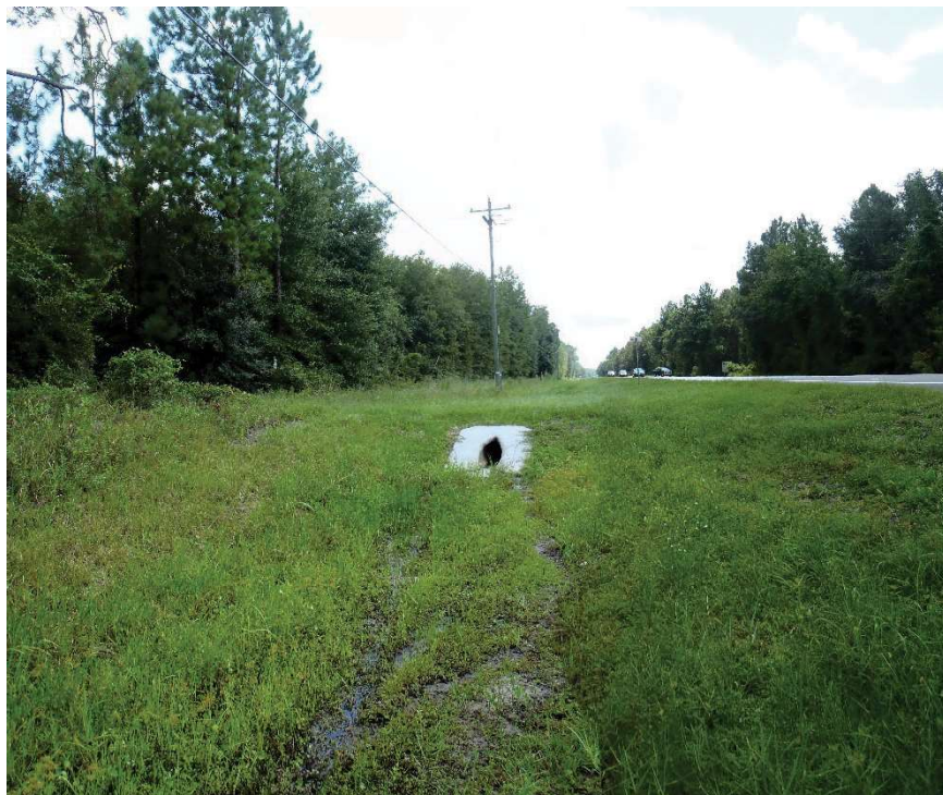
Photo 143. View of Physical Feature: Culvert as seen looking south from GPS location 1038 (Frames 1781-1782; 08/26/15).
