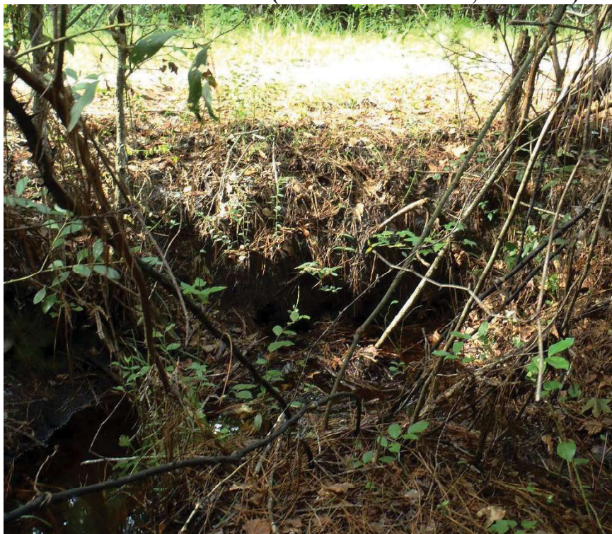
Photo 177. View of Physical Feature: Culvert located on south side of road at GPS location 1308 (Frame 1840; 08/27/15).
