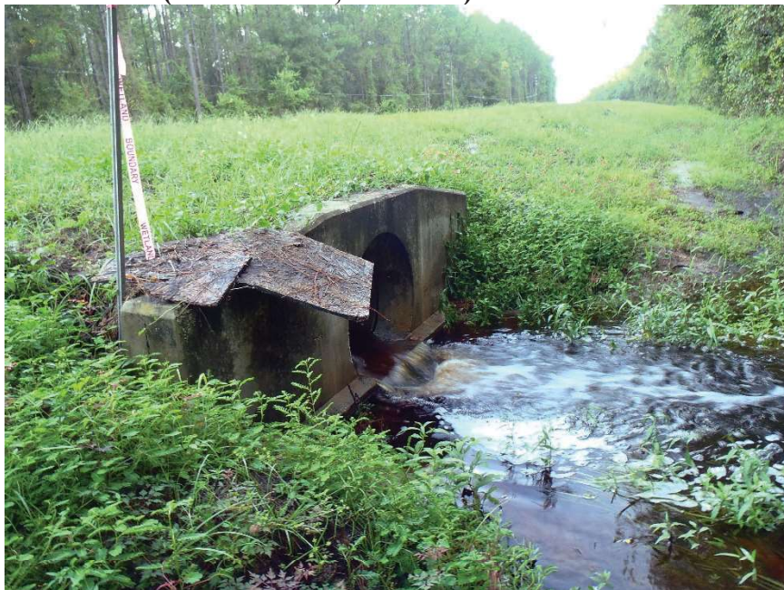
Photo 218. View of Physical Feature: Culvert located on east side of road as seen at GPS location 1697 (Frame 1893; 08/31/15).
