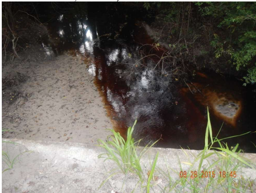
Photo 197. View to east (upstream) of major branch of Rocky Creek at culvert located at GPS location 1518 (Frame 7414; 08/28/15).
