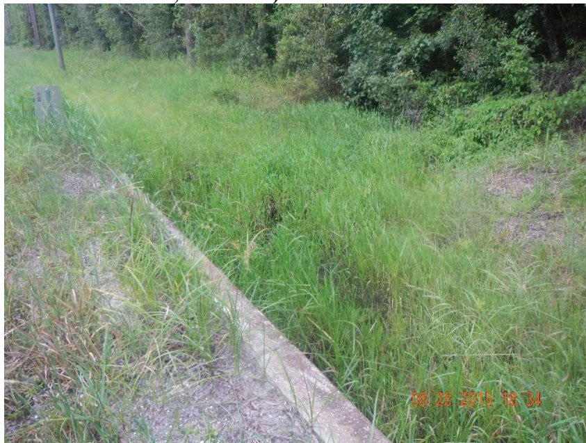
Photo 193. Rocky Creek: view to south of box culverts on west side of CR 231 at GPS location 1516 (Frame 7408; 08/28/15).
