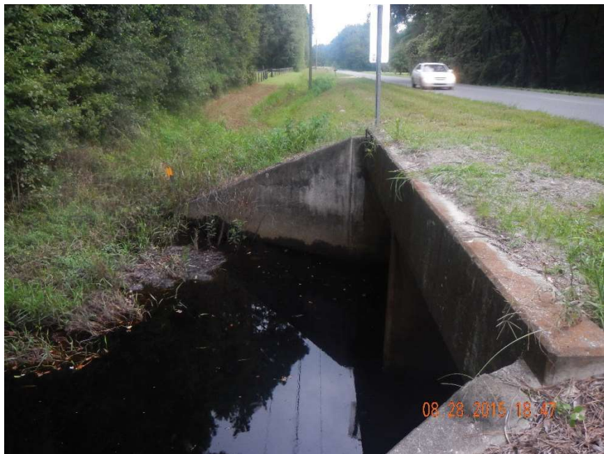
Photo 200. Rocky Creek: view to north along CR 231 of west side of box culverts located at GPS location 1518 (Frame 7420; 08/28/15).
