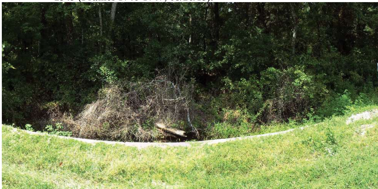
Photo 129. View of Physical Feature: Culvert as seen looking west from GPS location 2344 (Frames 1748-1749; 08/26/15).
