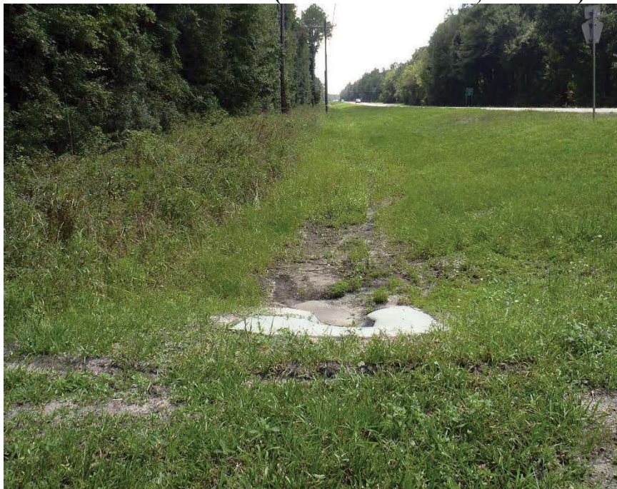
Photo 146. View of Physical Feature: Culvert as seen looking south from GPS location 1040 (Frame 1787; 08/26/15).
